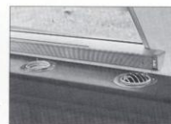
Air conditioning alternate location on wheelhouse has two adjustable grilles.
